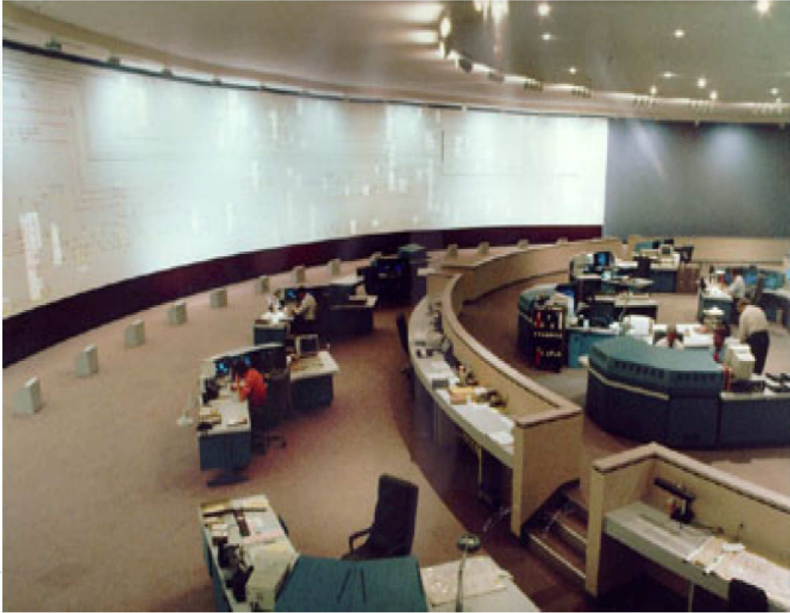
Figure 2.10: SCADA master control station [6]
